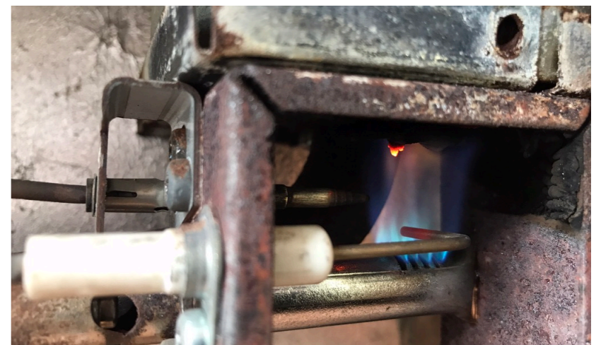
Burner, igniter and thermocouple are clean
