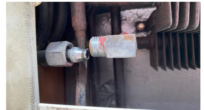
The gas pipe is now loose
